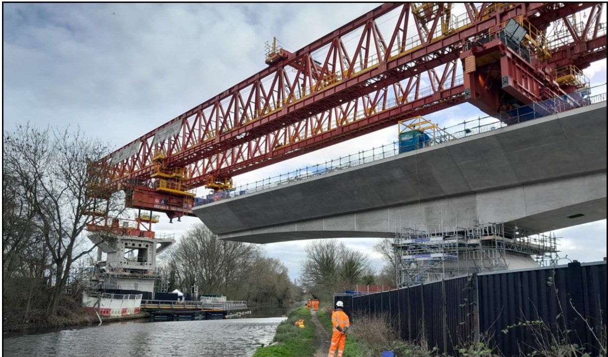
Aerial photo below shows the remaining works to be completed on the Viaduct as it heads towards Dews Lane
